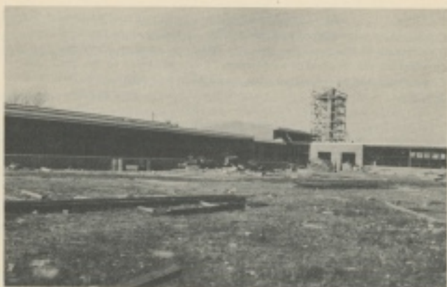
New Wildwood Elementary School , now under construction 14 classrooms, all purpose room, library, etc.
